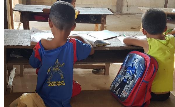
Superheroes of Laos – Children are staying in a partially damaged building with hazardous structural damages in Savanakhet. Photo credit: Tara I.M., Plan International Australia.
