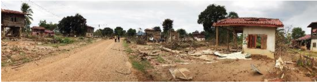
Panorama view of affected houses in Sanamxay District of Attapeu province. ©UN-HABITAT
