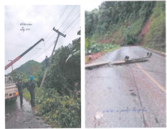
Example of damaged distribution grids
