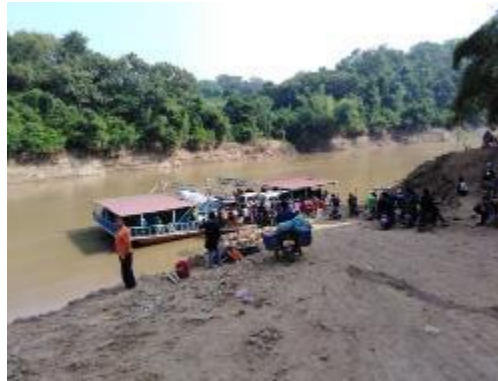
Nam Xeuang Bridge Damaged of approach slab (photo on 5 October 2018)
